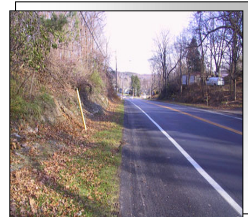
The existing deep scoured ditches along the steep roadside grade were replaced with closed systems
